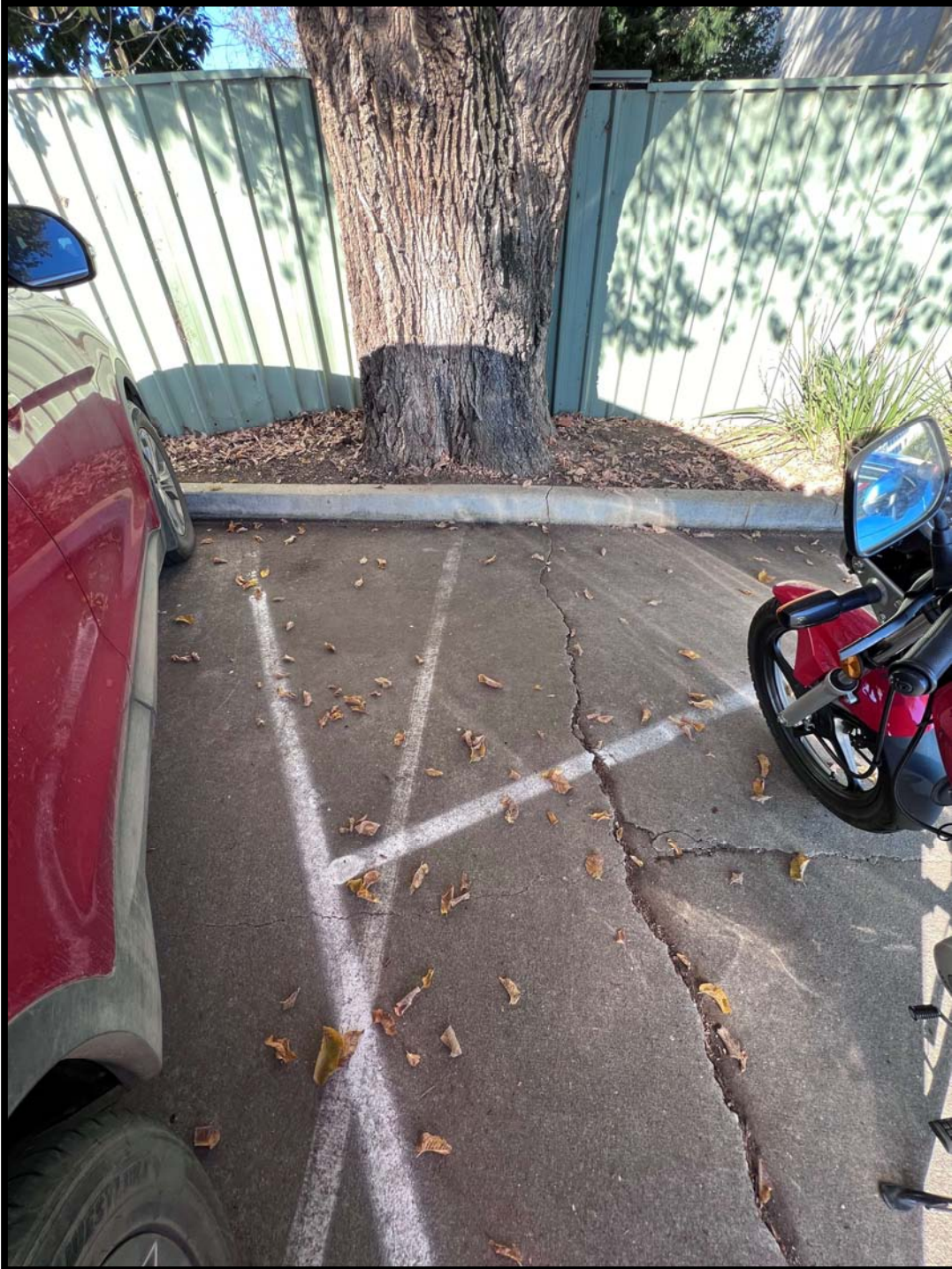
Exhibit 6 – The tree’s northern root plate has been “sealed” by the construction of a concrete surfaced car park. The cracking and displacement of the concrete surface (and kerb) is probably attributable to the continued growth of the tree’s structural roots.
